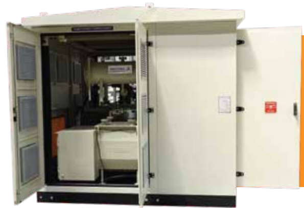
CSS Transformer Compartment
